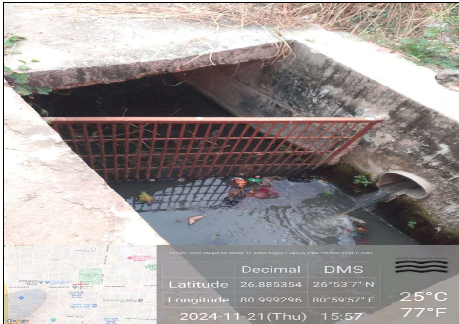
Indra Nagar Near Jama Masjid Road, Nala Mesh Filtration
